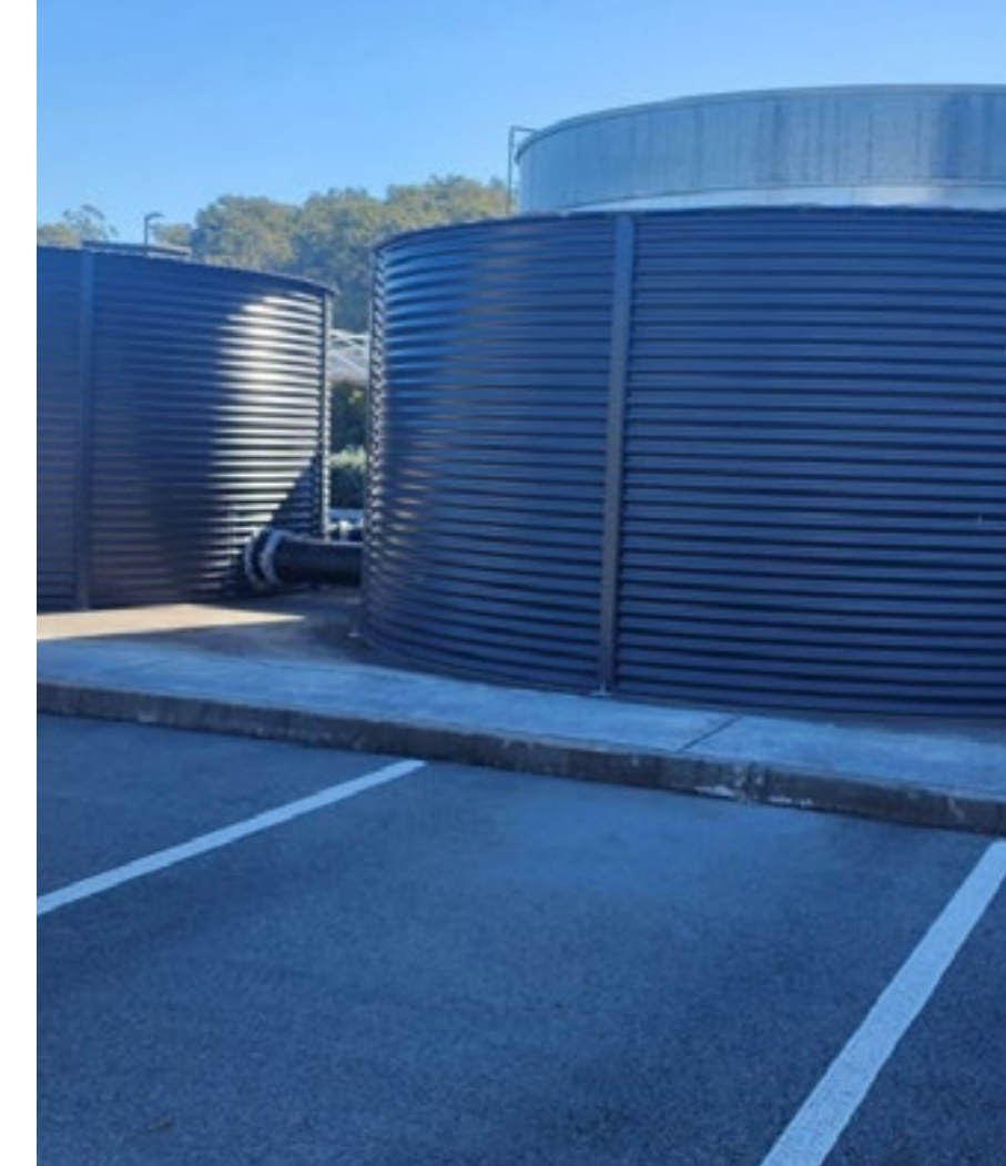
Reward Hospitality, Australia, rainwater collection
